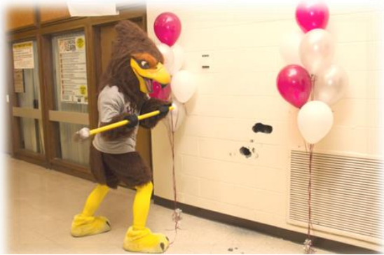
Hemingway Hawk does his part for the Cooper renovation project, striking the first blows in the demolition phase.
